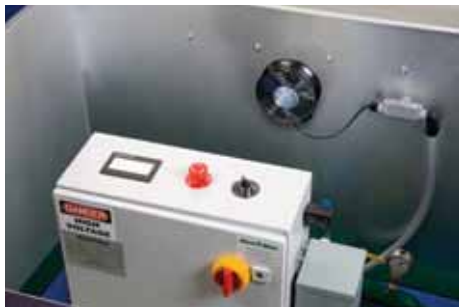
Interior of Low Profile Pump Station (LP)
