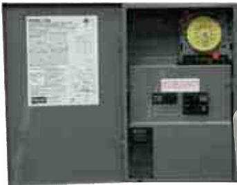
230v Control Panel
